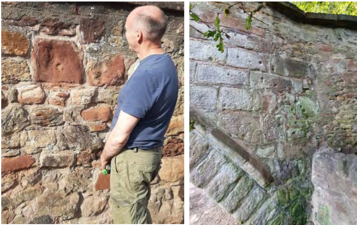
Figure 33 – Whereas shot holes are easily found on the buttresses the Nungate Bridge (right) finding similar evidence of war damage in the Friary precinct wall is difficult to spot as much of the stonework has been covered over with mortar or replaced. Here potential shot hole has been found in the south wall of the precinct, an area which witnessed heavy fighting on 10 th Oct 1548
