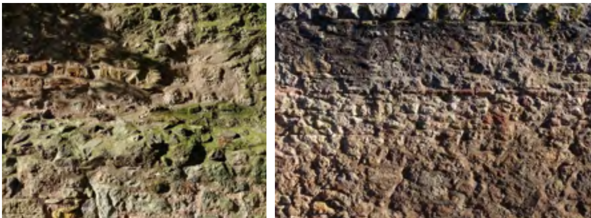
Figure 29 - By studying the layering of the stonework in various sections of the wall it should be possible to work out the history of each wall section.
